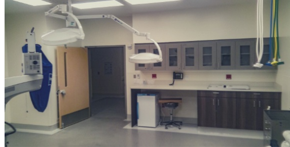
BCH CMC MOB 2 PREMIER EYE SURGERY CENTER TI Location: Lafayette Architect: Boulder Associates
